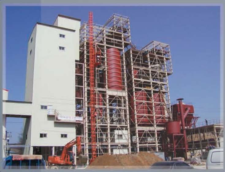
Dry Mortar Plant (대구)
